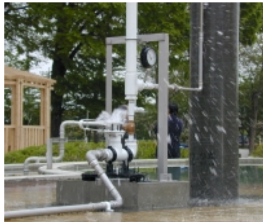
Fig. 28 Water Hammer Pump in Operation
